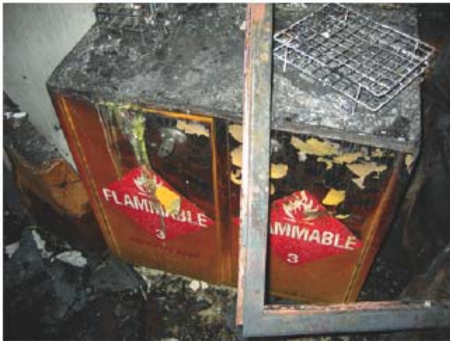
Fire burnt the exterior of the storage cabinet
